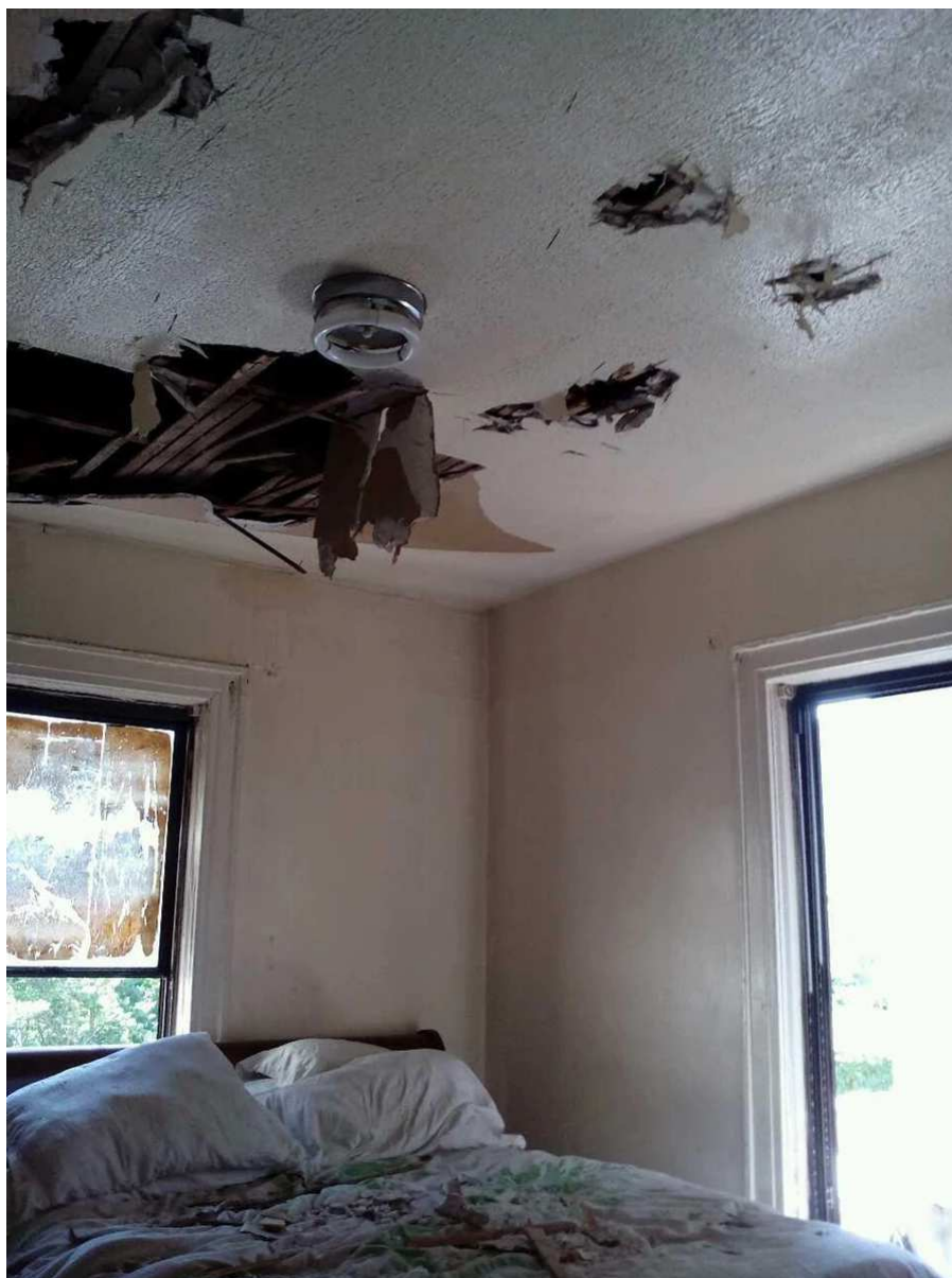
Richards' bed was covered in plaster after her landlord allegedly destroyed her ceiling with a sledgehammer. Photo Credit: Michelle Richards
