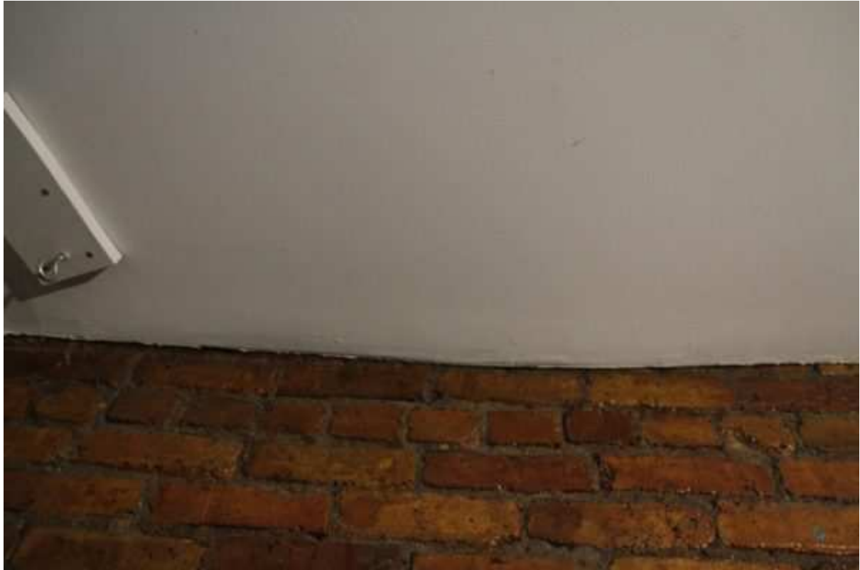
Above and below, photos of the ceiling at 159 Stanton St, that was deemed “dislodged and in danger of collapse” by the Department of Buildings, leading to an emergency vacate order.
