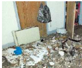
Damage from Shawn Dahl’s apartment, which she claims was caused by irresponsible repairs in the building.
